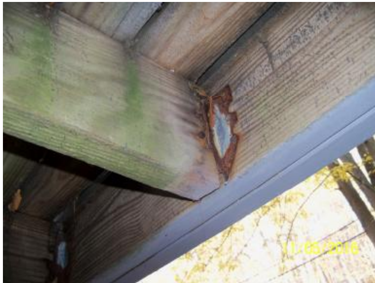
Figure 5. The bottom of this joist hanger has rusted away.
