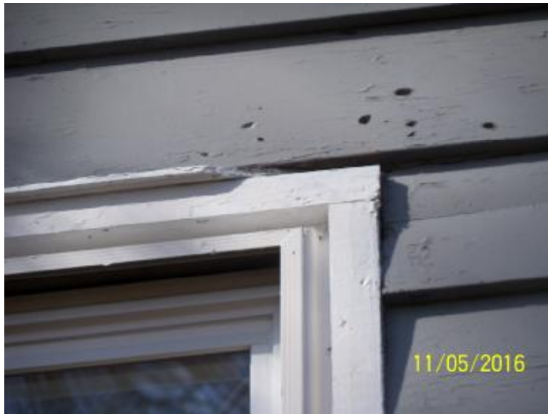
Figure 1. Damaged drip cap; also note the woodpecker damage.
