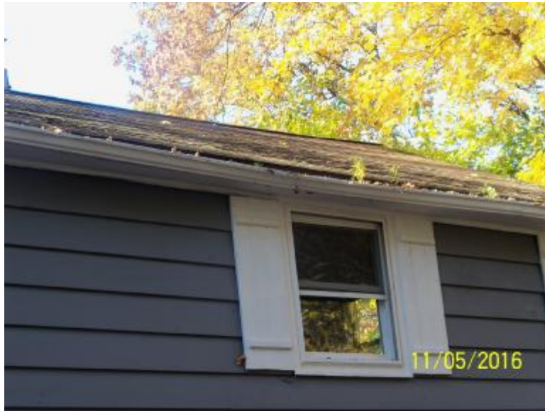
Figure 2. Sagging gutter at front right side. Also note the leaves that are clogging the gutters.
